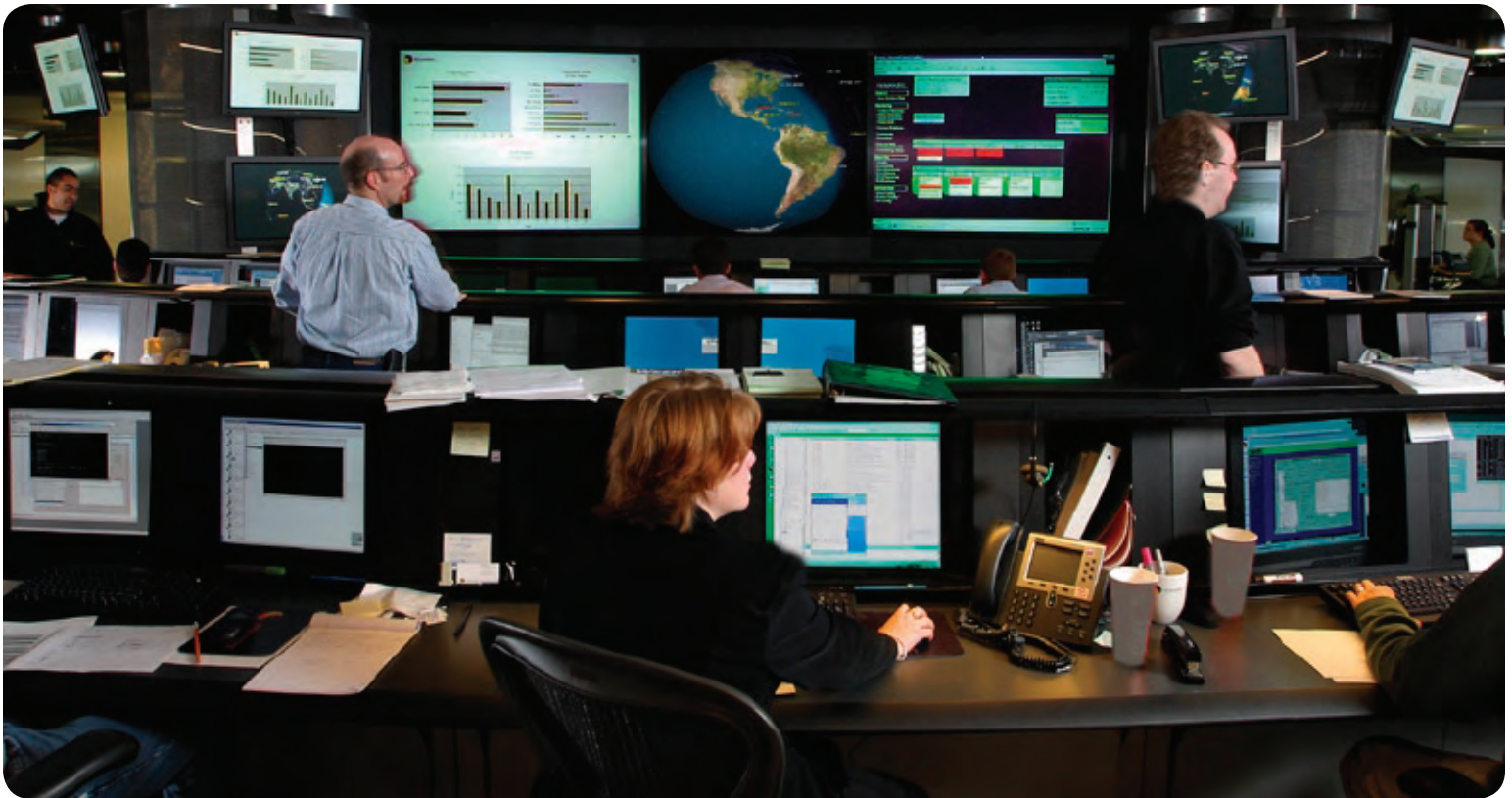
One of four global Symantec Security Operations Centers staffed with Symantec security experts and certified against ISO 27001 and SAS70 Type II specifications
